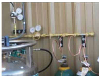
Liquid Oxygen Manifold & H-Tank
